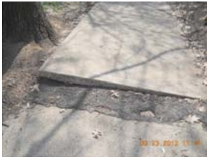
Figure 2-32: Severe Vertical Elevation as Obstruction
