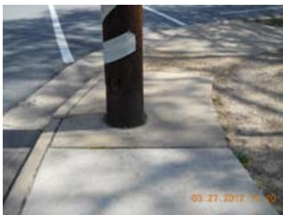
Figure 2-29: Utility Pole as Obstruction
