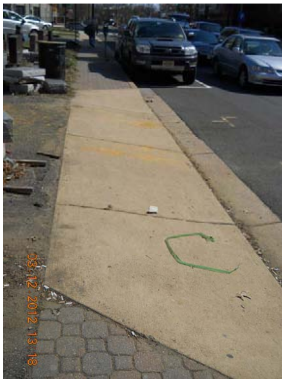
Figure 1-20: Inaccessible Driveway Crossing with Severe Cross Slope
