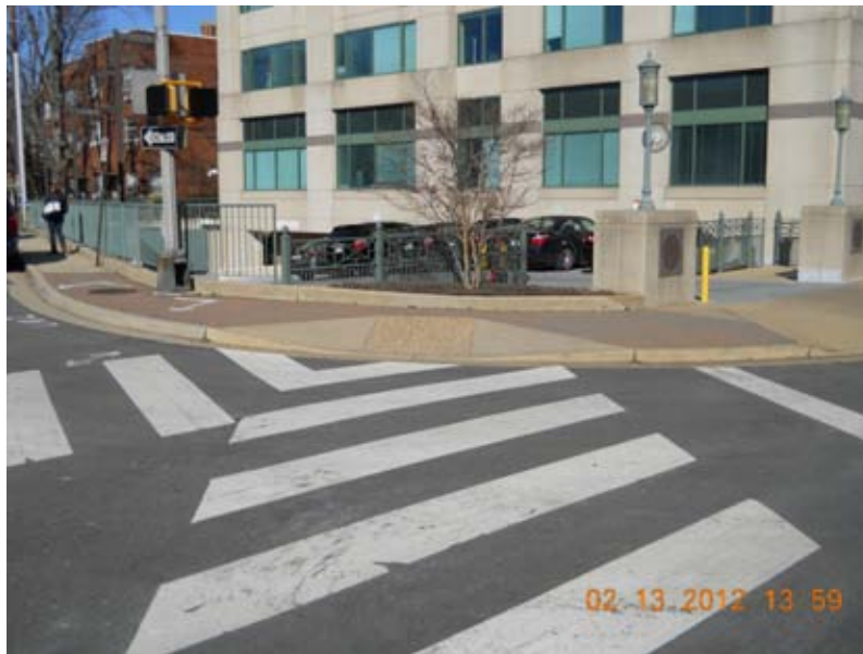
Figure 1-5: Diagonal Curb Ramp with Room to Maneuver Within the Crosswalk in Arlington, VA
