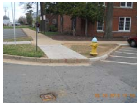
Figure 2-54: Missing Curb Ramp Example
