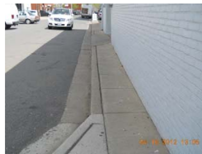
Figure 2-26: Sidewalk Less Than 36\"
