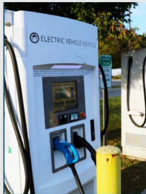
Figure 13: EV charging station (MDOT).
