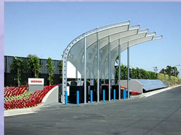
Honda hydrogen production and fueling station for fuel cell vehicles in Torrance, CA
