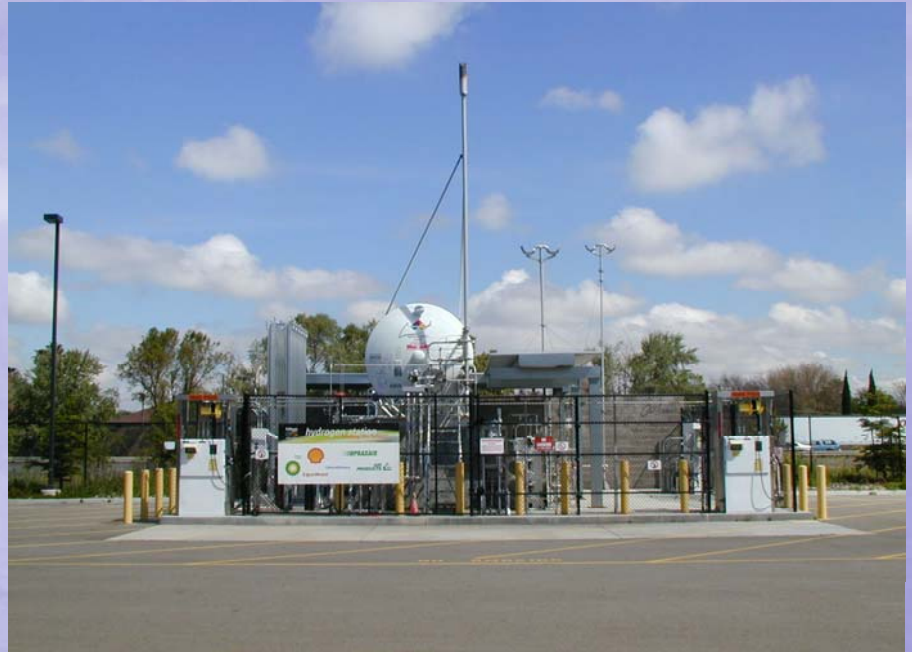
California Fuel Cell Partnership hydrogen fueling station
