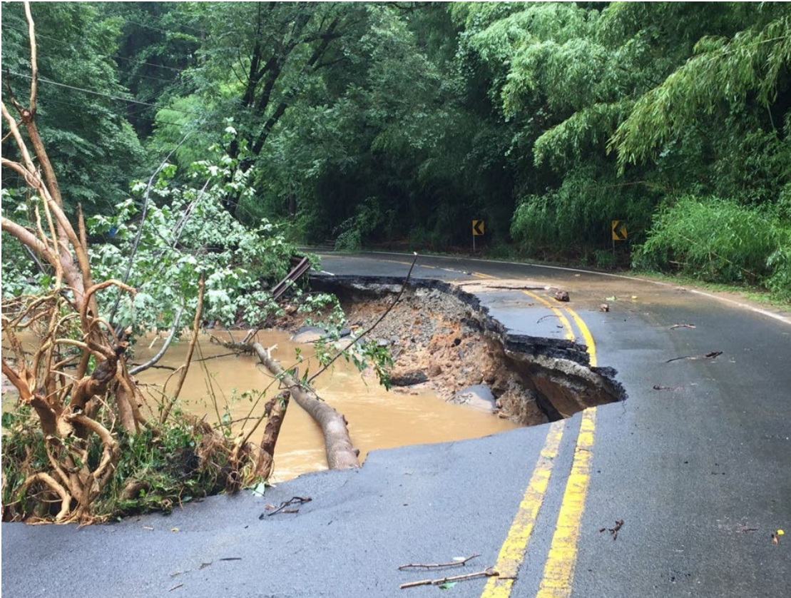
Damage along Kirby Road from the July 8, 2019 Flooding Event. Fairfax County PD
