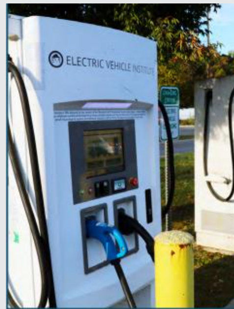
Figure 13: EV charging station (MDOT).
