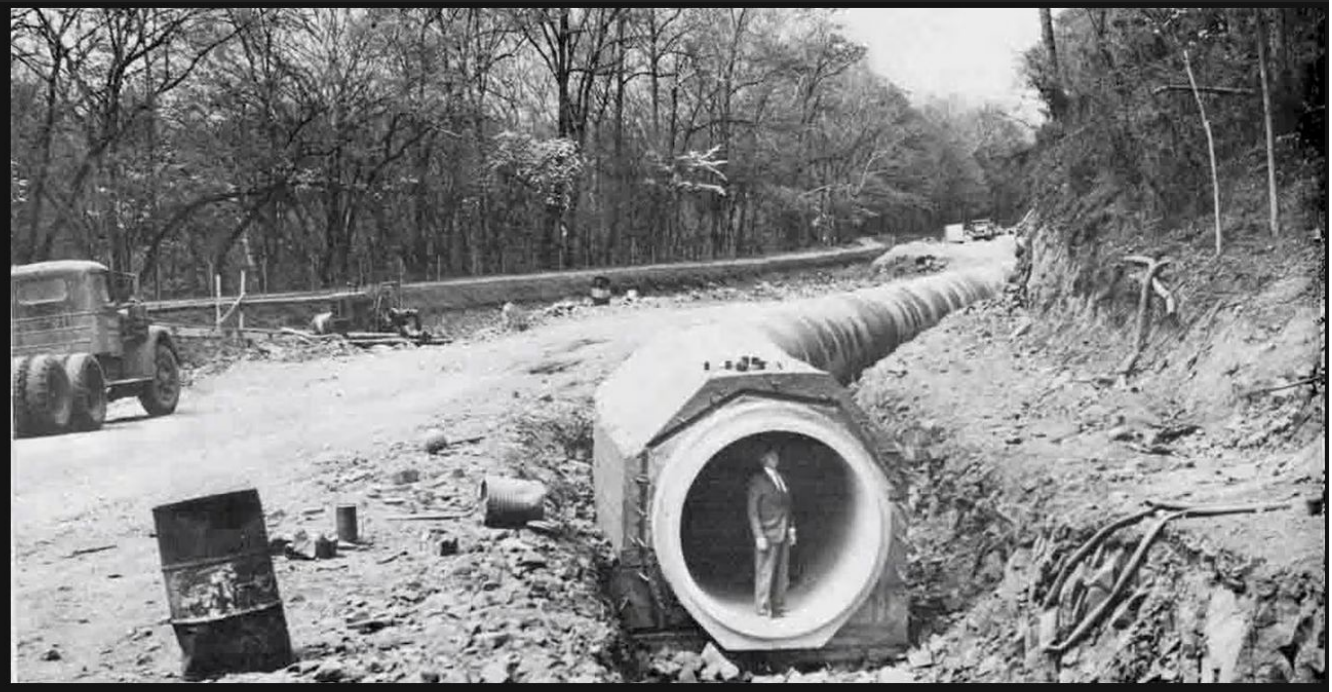
Construction in the 1960s of the sewer line now known as the Potomac Interceptor. (D.C. Water)
