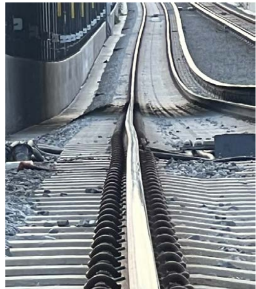
Figure 3. Heat kink on WMATA’s Blue and Yellow rail service line on July 14, 2024. Source: DCNewsNow, 2024.
