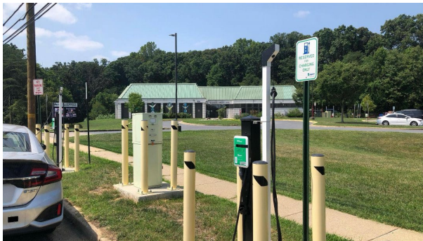
EV charging stations at Bladensburg Community Center (Source: Town of Bladensburg )
