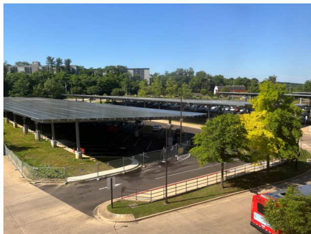
Solar Carports at the Naylor Road Metrorail Station’s Parking Lot (Pierre Gaunard/TPB)
