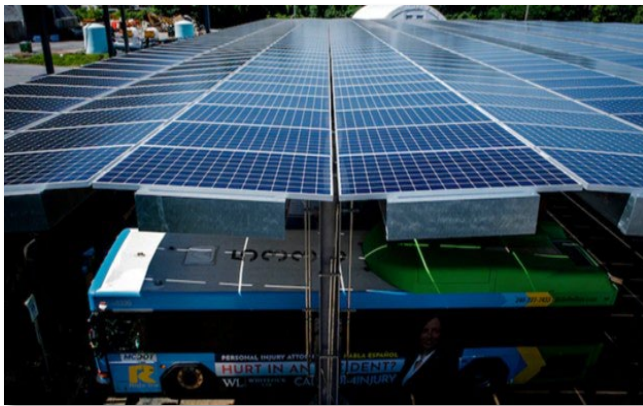
Brookville Smart Energy Depot Bus Parking Under Solar Canopy (AlphaStruxure and Montgomery County, MD/USDOT - FHWA)
