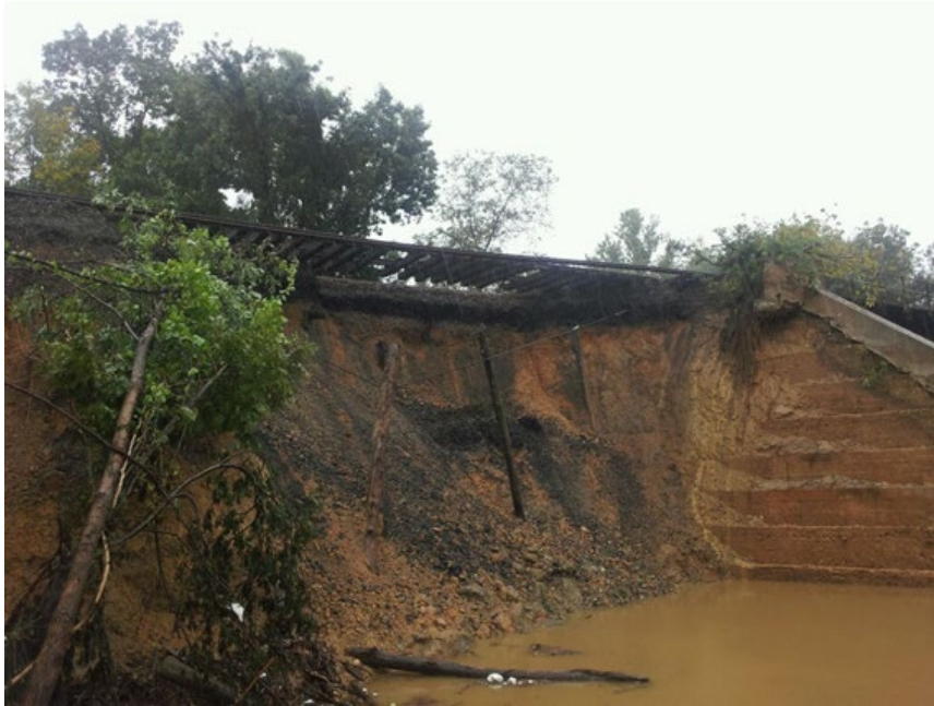
VRE Tracks Washed Out near Springfield, VA Due to Flooding in September 2011. (VRE)
