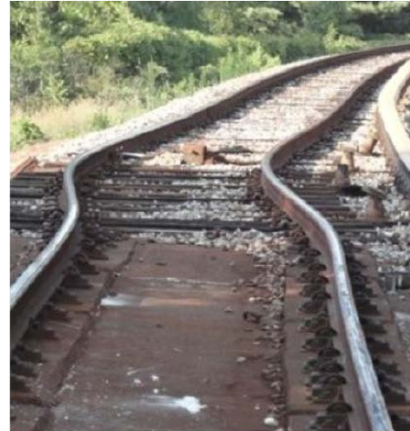
Figure 11. Buckling Caused by Heat Wave on Metro Green Line. Source: Washington Post in the COG Adaptation Summary.
