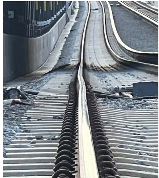
Figure 8. Heat kink on WMATA’s Blue and Yellow rail service line on July 14, 2024. Source: DCNewsNow, 2024.
